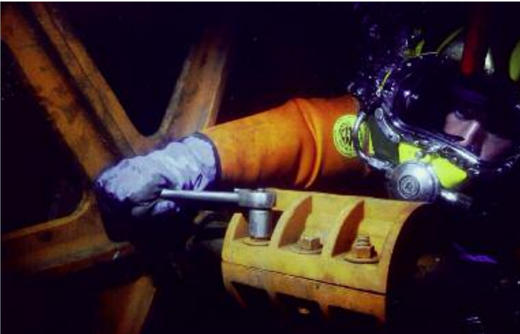
Our expert service technicians and certified divers will inspect and refurbish your traveling water screen for optimum performance.
